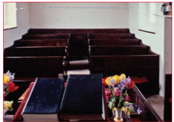
A survey of chapels in the late 1990s revealed the rarity of chapels with interior fittings that date from the 1860s and earlier. The best examples have been listed at grade II*. Penrose Bible Christian Chapel (1861) in St Ervan parish is such a survival of a small vernacular chapel with interior fittings including box pews. It has limited adaptability for new uses, and following a period of disuse it is now in the care of the Historic Chapels Trust. Photo © Eric Berry
