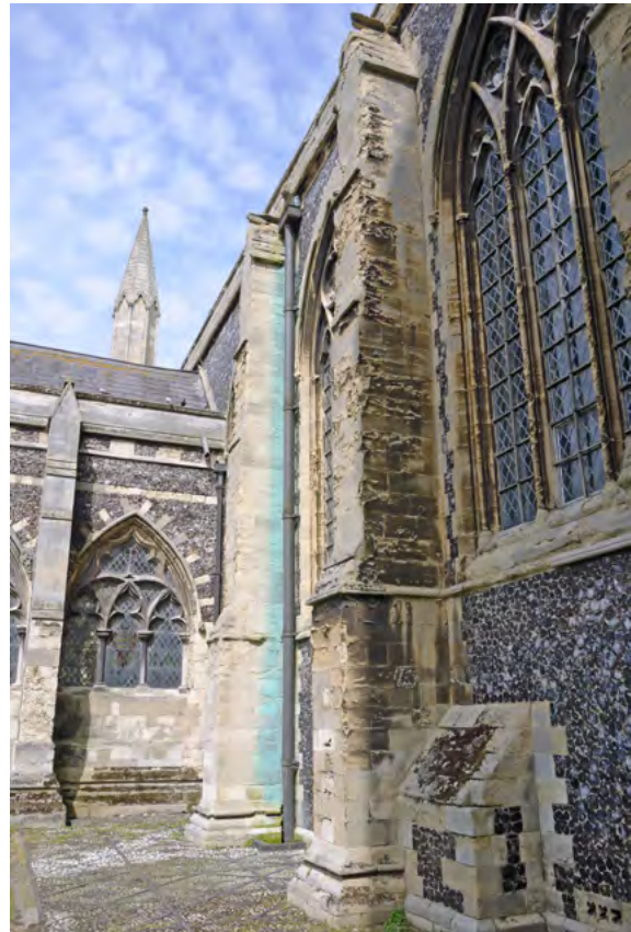
Damaged stonework in need of repair
