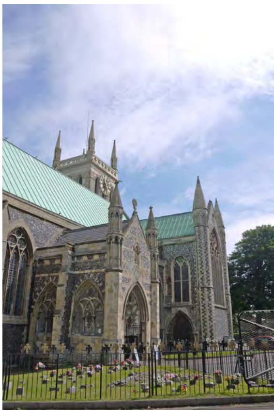
View of the south porch roof, which is soon to be repaired
