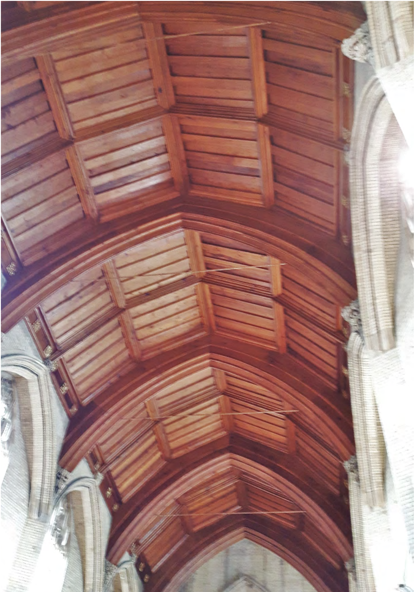
St Agatha's roof, which was rebuilt to Bidlake's original design following a fire in 1959
