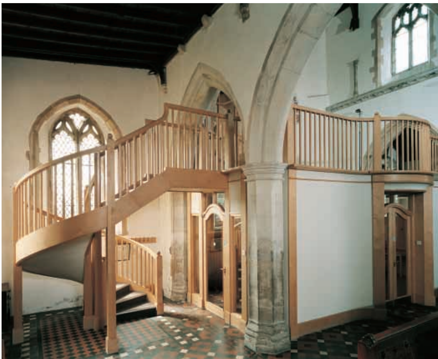
Figure 7 New facilities have been created here by enclosing the western bay of the nave and tower area.
