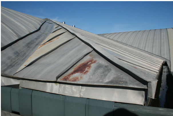
Figure 9: Discolouration of lead-rich terne-coated stainless steel
