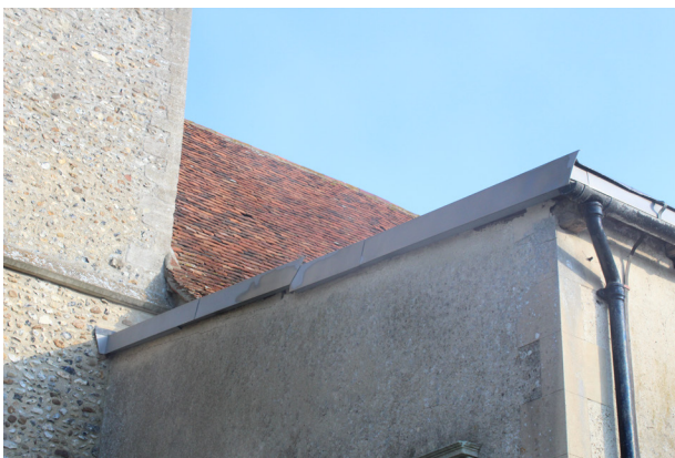
Figure 7: Straight verge fascia contrasts with uneven masonry
