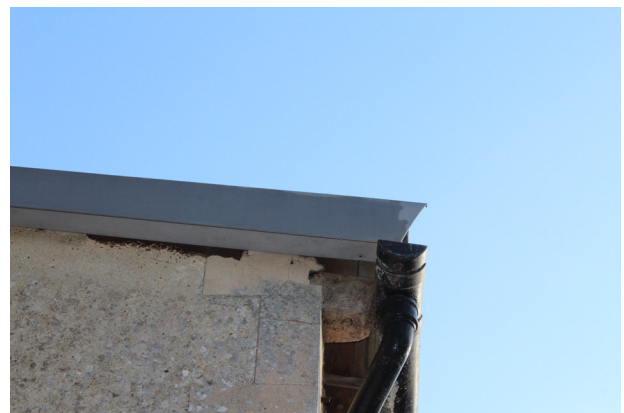
Figure 8: End of fascia with acute corner and incomplete closure
