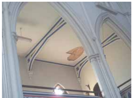
Effects of water penetration to south aisle of nave, 2006
