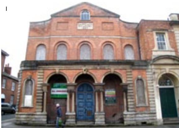
1 Vacancy and lack of regular maintenance make redundant buildings extremely vulnerable to decay and vandalism. © Sara Crofts.
